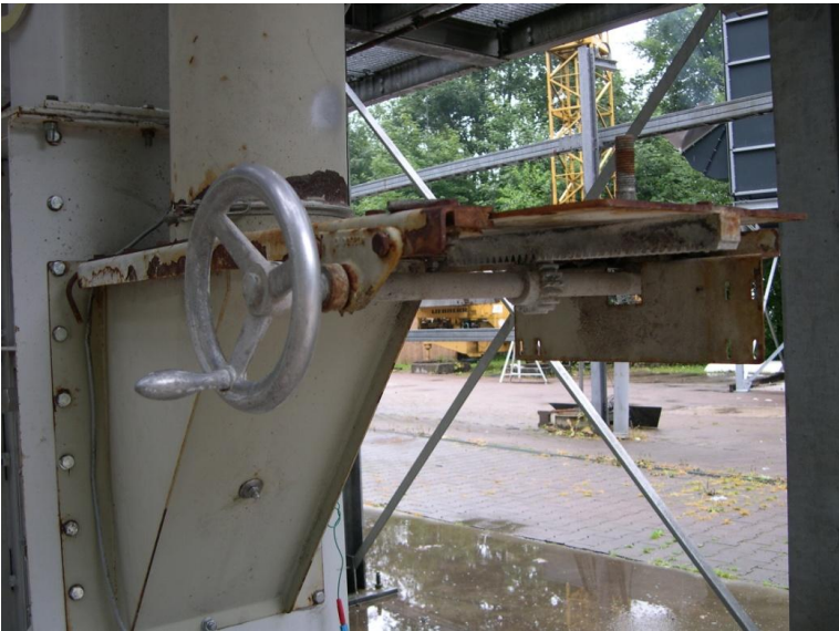
Figure A3: Gate valve at the elevator boot / down pipe
