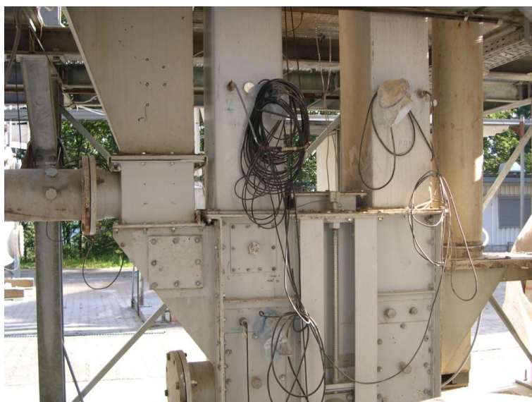
Figure A2: Elevator boot with inlet pipe (at the left side) and down pipe (at the right side)
