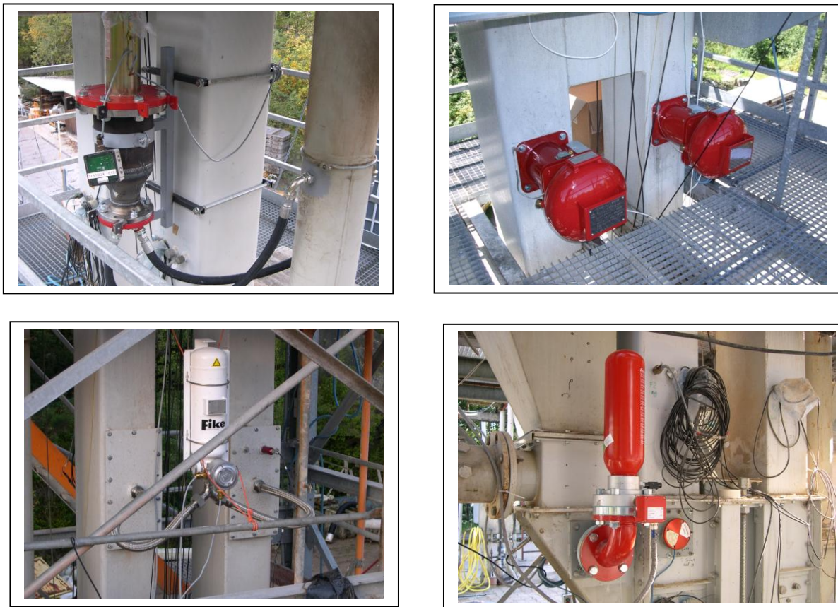
Figure 2: Bucket elevator with extinguishing agent containers from different manufacturers
