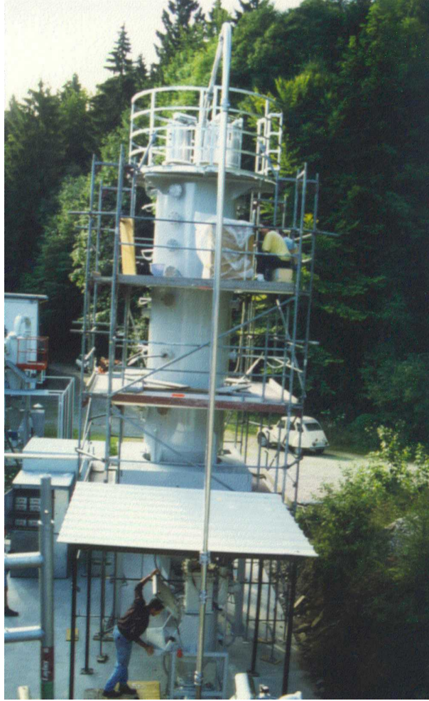
Figure 11: Photograph of the 12 m 3 -silo fed vertically pneumatically.
